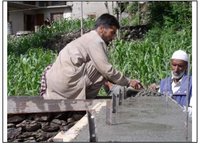
Installing MS angle and single rod connectors for roof structure anchoring in eave band
