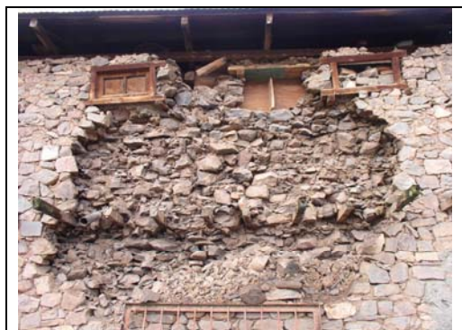
Delamination of UCR wall
