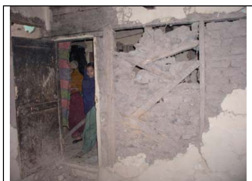
Damage to Dhajji wall infill
