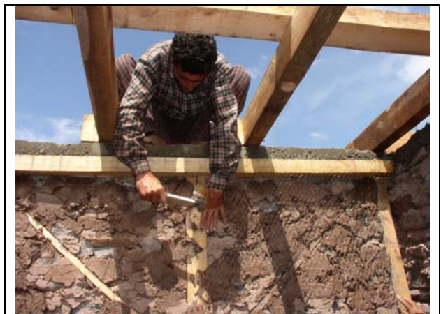
Chicken Wire Mesh confinement on Dhajji wall
