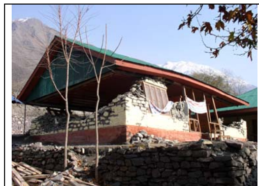
Collapse of UCR wall
