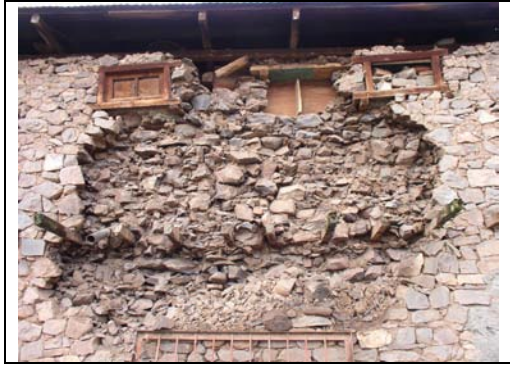
Delamination of UCR wall
