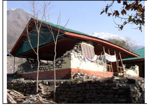
Collapse of UCR wall
