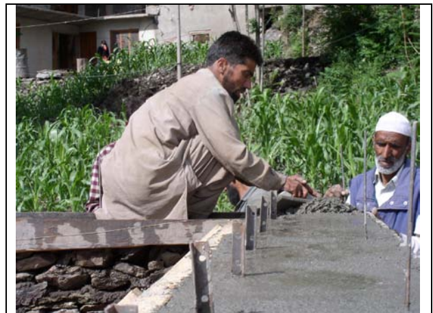
Installing MS angle and single rod connectors for roof structure anchoring in eave band
