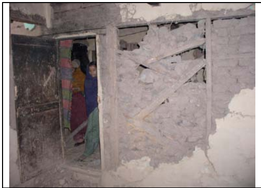
Damage to Dhajji wall infill
